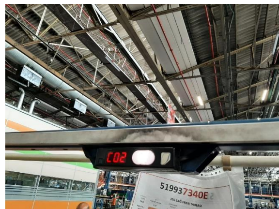
Figure 16. Pick to light device above each input container
