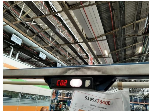
Figure 20. Pick to light device above each input container
